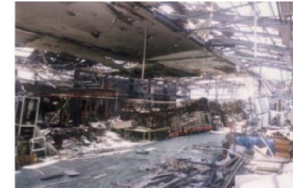
Condition of burned facilities
