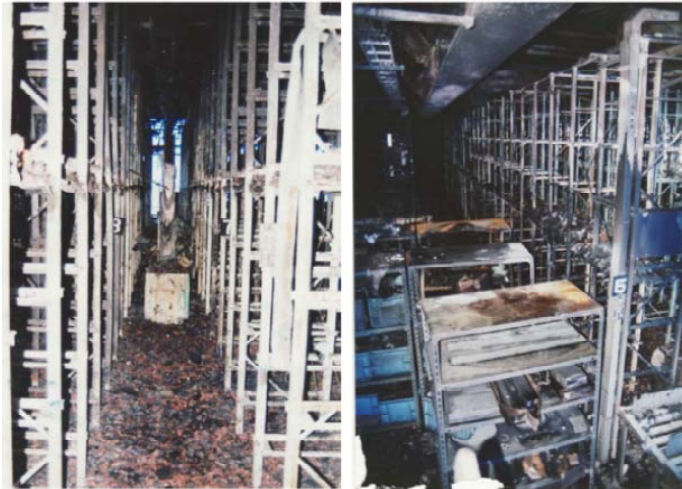
Conditions of damage in the warehouse area
