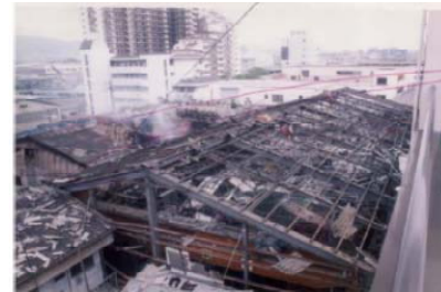
Roof blown off by the fire
